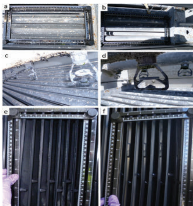
Figure 10: Surface condition evolution between the technical shutdown in November 2019 (left) and June 2020 (right) at Site G. a and b: View of the upper tubes (Point 3 on the schema in Figure 9); c and d: View of the spray ramps and a set of nozzles (Point 3 on the schema in Figure 9); e and f: View of the packing's trickle lamellas.
