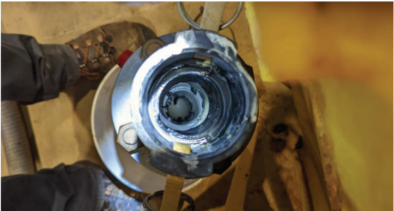
Figure 8: Swollen and degraded EPDM gasket in the polymer feed line that caused pump plugging and damage as pieces broke off
