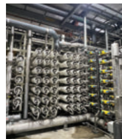
City of Santa Monica (California) Arcadia Water Treatment Plant retrofitted with flow-reversal reverse osmosis.
