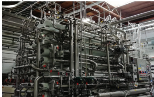
Figure 8: Additional valves and piping added to the RO recovery unit.
