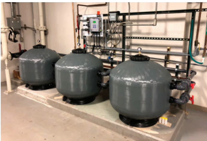
A commercial installation of contact chambers that hold the Sphagnum moss-based treatment products.
